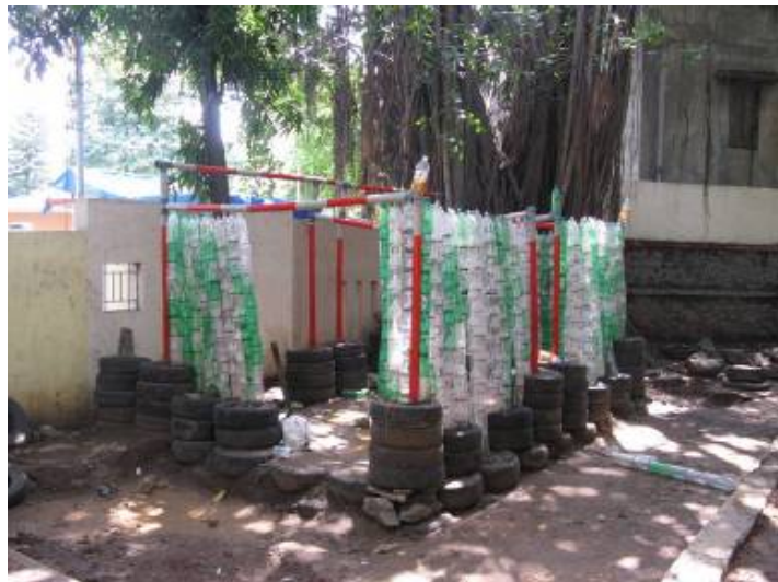
Frame collapses due to welled up tarp..
